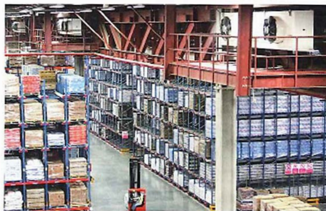
thermofin air coolers in a large distribution centre in Saudi Arabia
